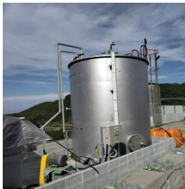
Asphalt Storage Tank
