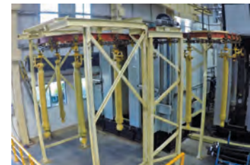
Automated Painting System (Seamless Integration with Assembly & Testing)
